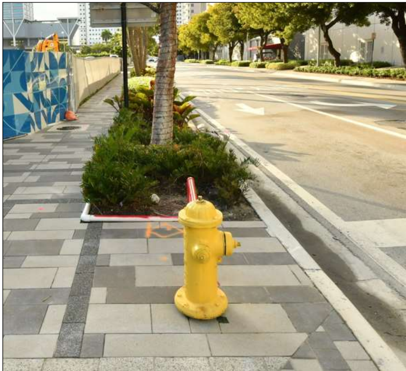
EXISTING UTILITY – FIRE HYDRANT
