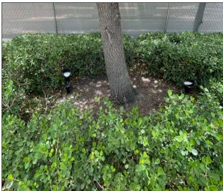
EXISTING UTILITY – LANDSCAPE LIGHTING
