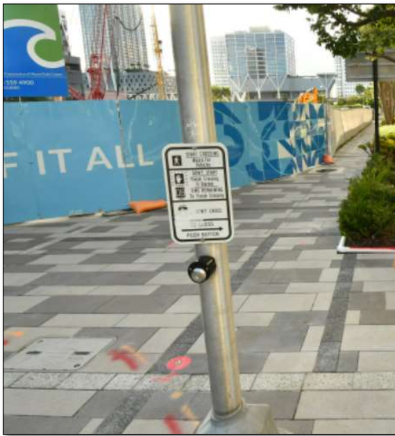
EXISTING UTILITY – PEDESTRIAN CROSSWALK SIGNAL
