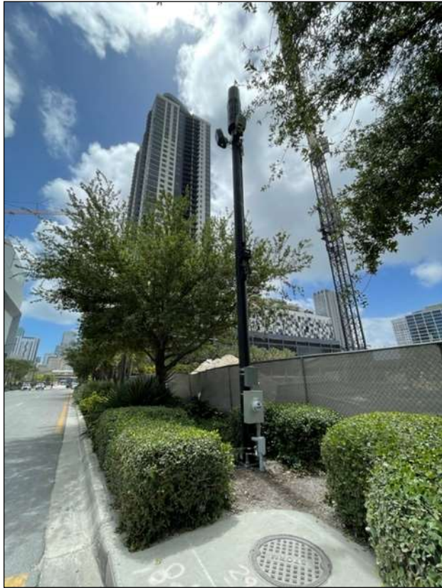
EXISTING UTILITY – 5G TOWER
